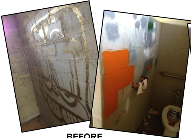
BEFORE Joyce Park Restrooms
